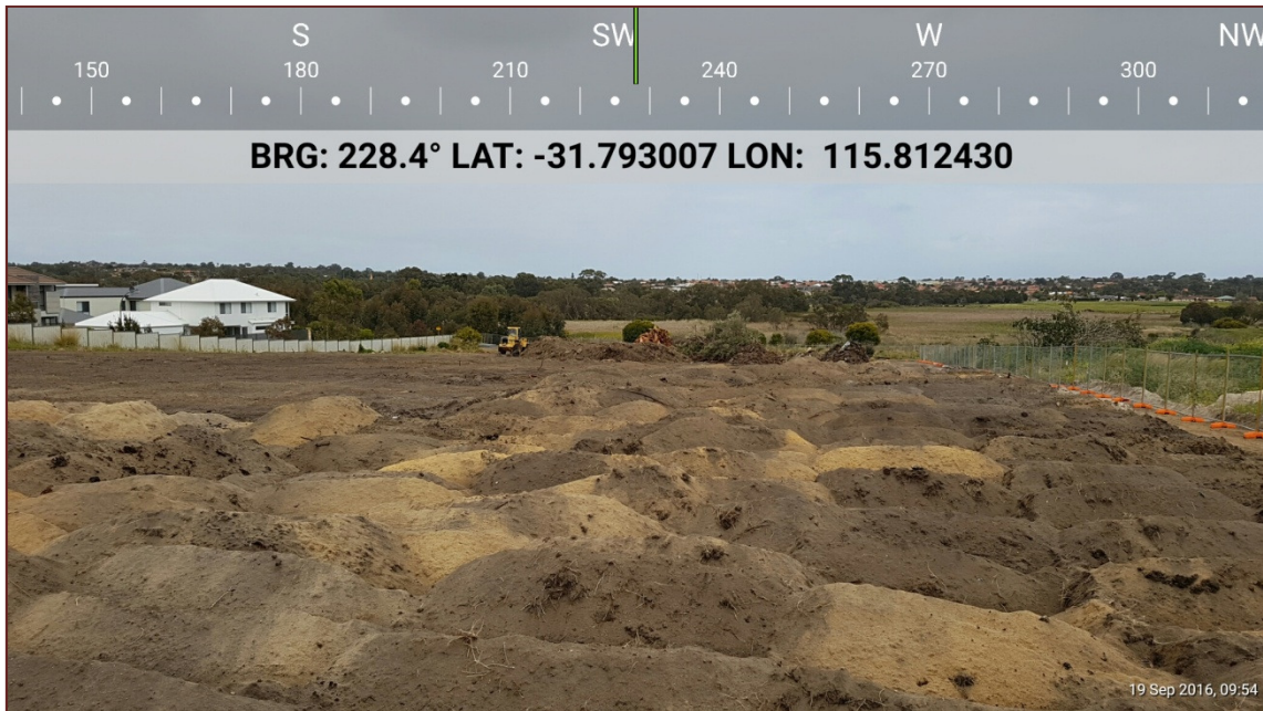
Plate 9: Photo Point 9: Excluded from classification under Clause 2.2.3.2 (e) of AS 3959–2009 within the project area
